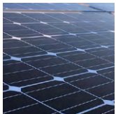
Solar panels mounted on shedded roof
